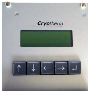
Level Control Device
